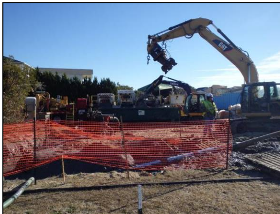
12" Fusible PVC® pipe ready for hydrotest and connection on Sunset Island side
